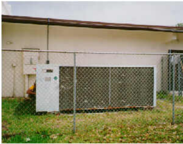
Figure 3. Forty-ton air cooled liquid chiller.
