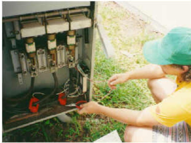
Figure 5. Stephen Barkaszi installs watt-hour transducers on the facility chiller to record electrical consumption.
