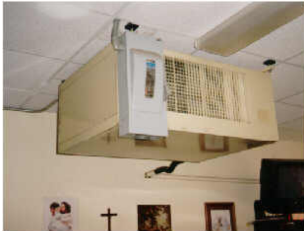
Figure 4. Ceiling mounted classroom air handler. Above acoustic tiles is R-19 insulation. Chilled water lines are located in roof plenum above insulation.
